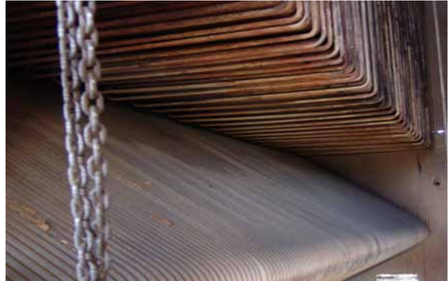
Furnace After TIFI® Treatment
