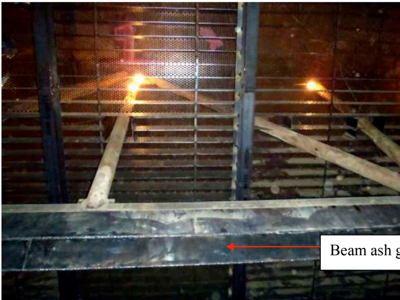
Figure 9: GSG shown below center truss with ash guard on lower truss beam
