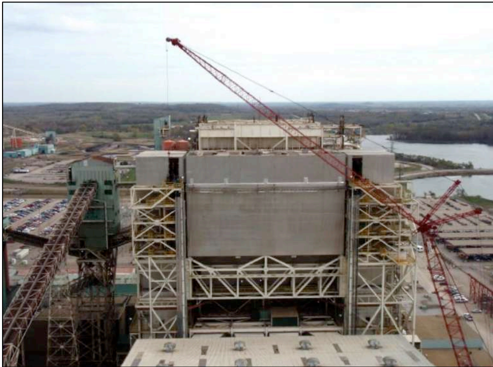
Figure 10: SCR crane and hood openings for material transport
