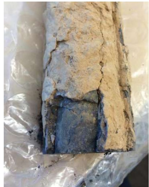
Figure 6. Severe chloride induced corrosion
