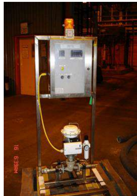
Figure 3. Corrosion Control Panel and Air Valve
