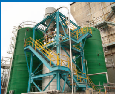
Urea solution storage tank
